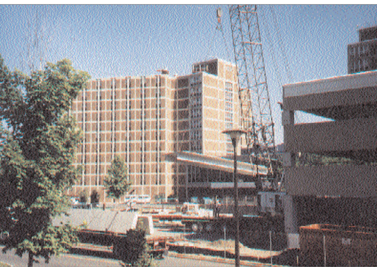
A crane lifts a prefabricated section of concrete floor into place at the new parking garage serving the Travers/Wolfe residential towers.
